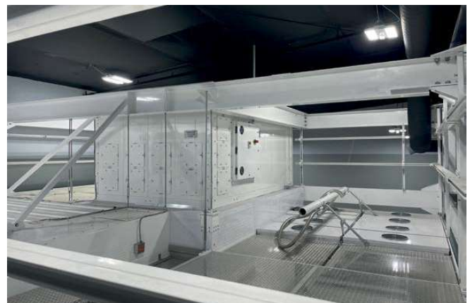
Figure 4: Walkable modular flush ceiling with plenum, recirculating AHU, sprinkler main and FFU All photos courtesy of Nortek Air Solutions CleanSpace.
