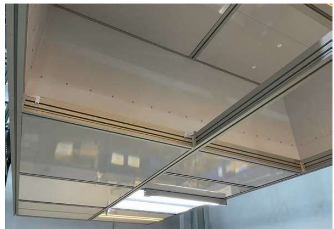
Figure 2: T Grid stick-built assembly with amber LED track lighting
